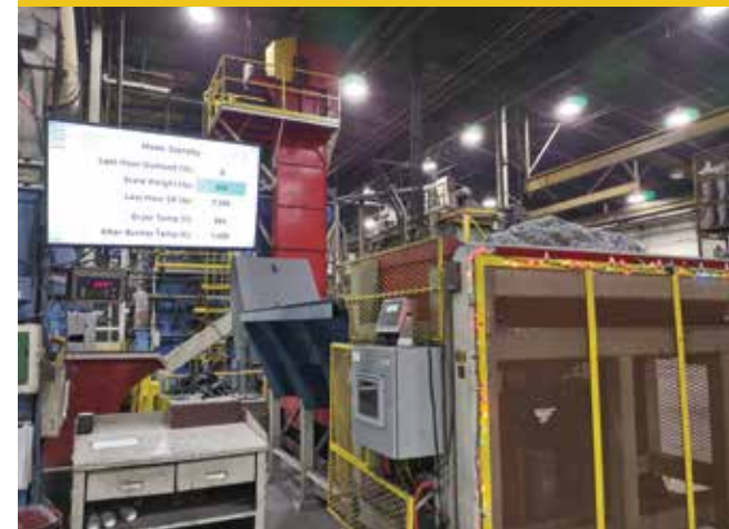
Mercury recycles aluminum machining chips into its metal for casting. There is a limit on how many pounds per hour can be processed, so the company put in a detailed data collection system to monitor and prevent them from exceeding their hourly rate.
